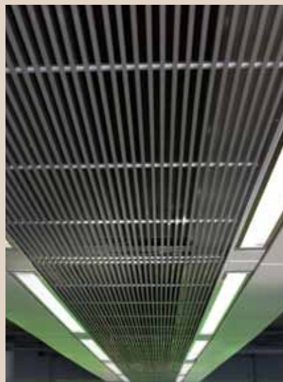
Charles H. Townes Center for Science at Furman University uses an energy-efficient cooling system using chilled beams, a technology widely used in Europe. At the time of construction in 2009, there were only two such cooling systems in use in the United States.
