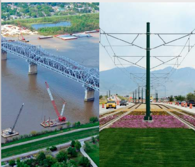
2013 Grand Award Winner Huey P. Long Bridge Widening (Main Span Superstructure) | Jefferson Parish, LA | Massman – Traylor – IHI, A Joint Venture (MTI)
