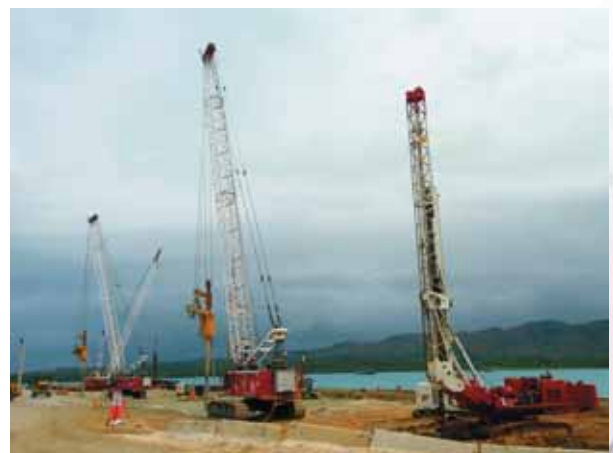
Project P204, Apra Harbor Wharf Improvements Phase 1, Naval Base, Guam Healy Tibbitts Builders, Inc. (Guam MACC Builders, A JV partner)
