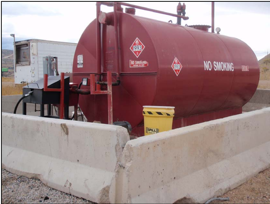
PHOTO #3 - 6,000 Gallon Diesel AST – Spill Kit, Example Labeling
