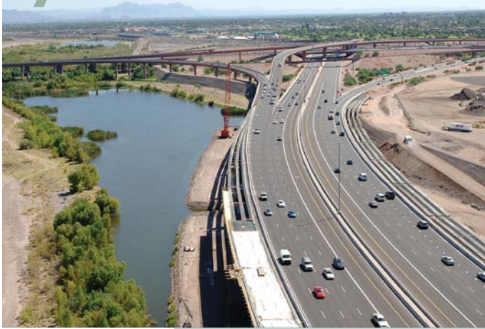
SR 202L Red Mountain Freeway | Design-Build | Phoenix, AZ | Kiewit/Sundt, a Joint Venture
